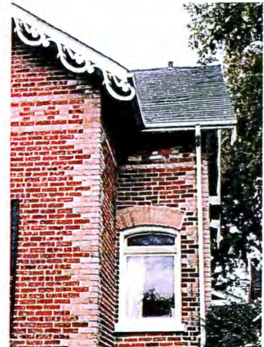
With occasional maintenance, the wood “gingerbread” trim and windows have lasted about 130 years. So far.
