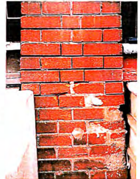
Progressive deterioration: Rainwater splashing on the porch and steps eroded the mortar. That let increasing amounts of water into the bricks and mortar below, and they are spalling and washing away, letting in even more moisture.
