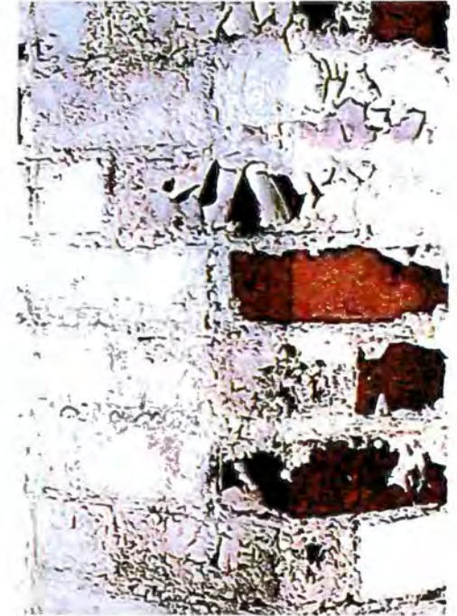
Non-breathing paint on brick. The vapour pressure of moisture in the brick blisters the paint, when it is able. If the paint adheres strongly, the pressure causes the brick surface to spall off, along with the paint, as seen in the centre of the picture. This lets in even more moisture, and the problem grows.
