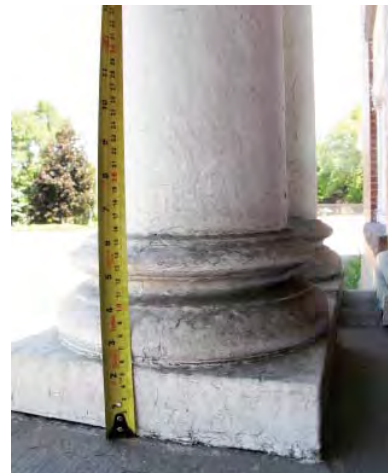
49. Investigate and document existing architectural elements prior to repair and restoration. (Source: ERA)
