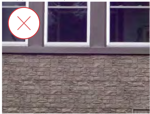
47. Artificial stone (seen here) or real stone cladding is not an appropriate material to use in Bolton. (Source: ERA)
