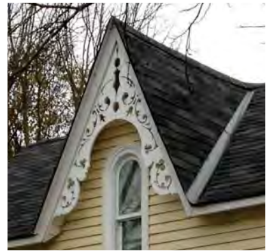
48. Maintain existing features such as this decorative bargeboard at 122 King Street East. This may require periodic repainting or refinishing. (Source: ERA)
