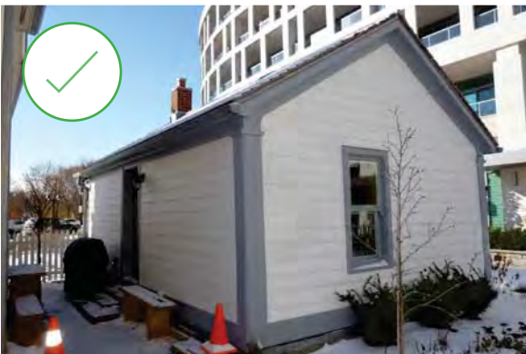
46. Hardie Board was used to repair one wall of this wood clad building in Bronte, Ontario. (Source: ERA)
