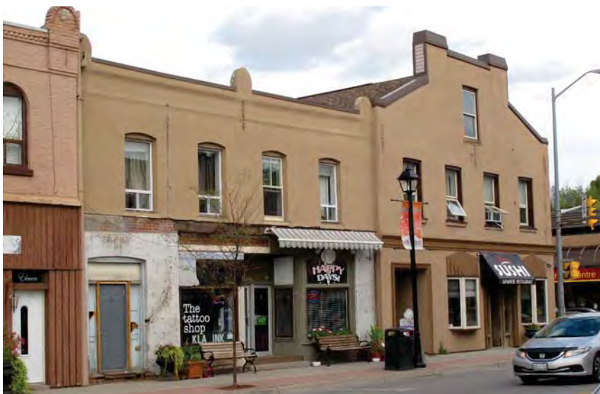
138. 5, 7 and 9 Queen Street North storefronts exposed following removal of modern cladding in August 2015, Bolton. (Source: Town of Caledon)
