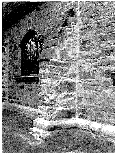
Figures 11 – 12: left – Christ Church, sketch plan, Registry of Stained Glass Windows in Canada, n.d.; right – buttress and foundation line viewed from the southeast (photo E. Tumak, July 2009).
