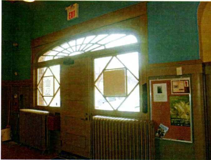
Interior view of main west-facing entrance showing elliptical fan light over five-panel door flanked by windows and panels (behind radiators); also shows wide casing, wainscoting and ledge.
